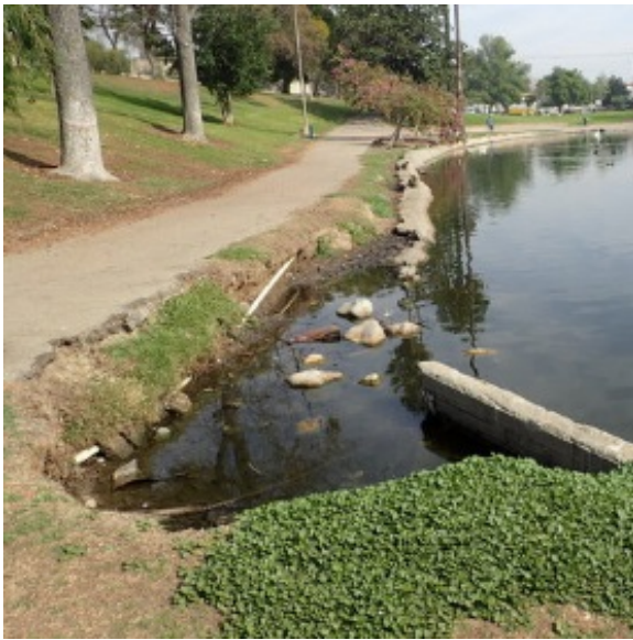
Figure 2-7-G. Lakeside Erosion Exposing Irrigation Lines Hollenbeck Park Lake Rehabilitation and Stormwater Management
