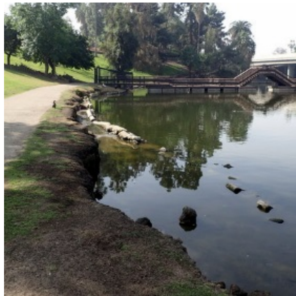
Figure 2-7-J. Lakeside Erosion Hollenbeck Park Lake Rehabilitation and Stormwater Management
