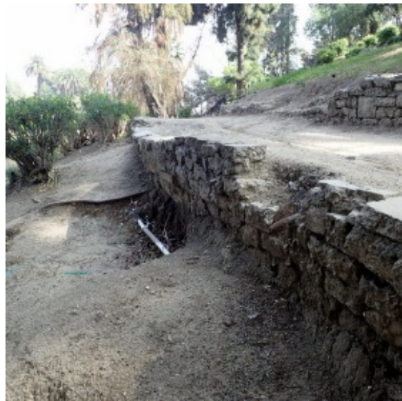
Figure 2-7-N. Hillside Erosion Exposing Irrigation Lines Hollenbeck Park Lake Rehabilitation and Stormwater Management
