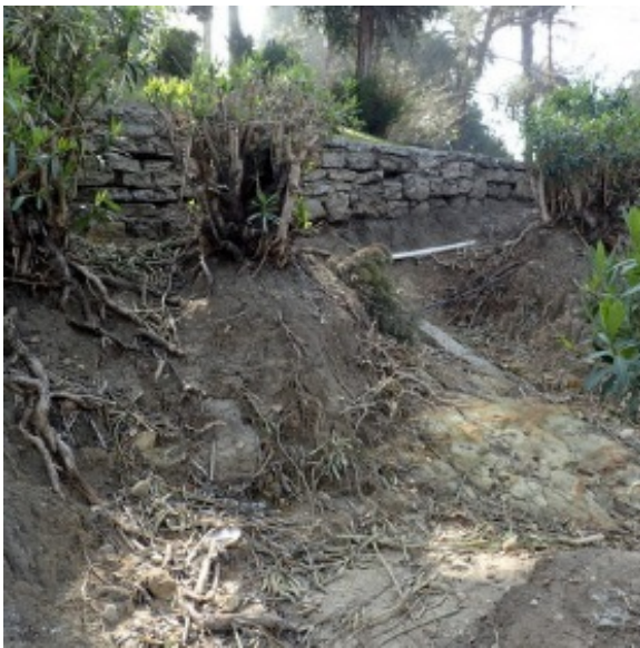
Figure 2-7-M. Hillside Erosion Exposing Irrigation Lines Hollenbeck Park Lake Rehabilitation and Stormwater Management
