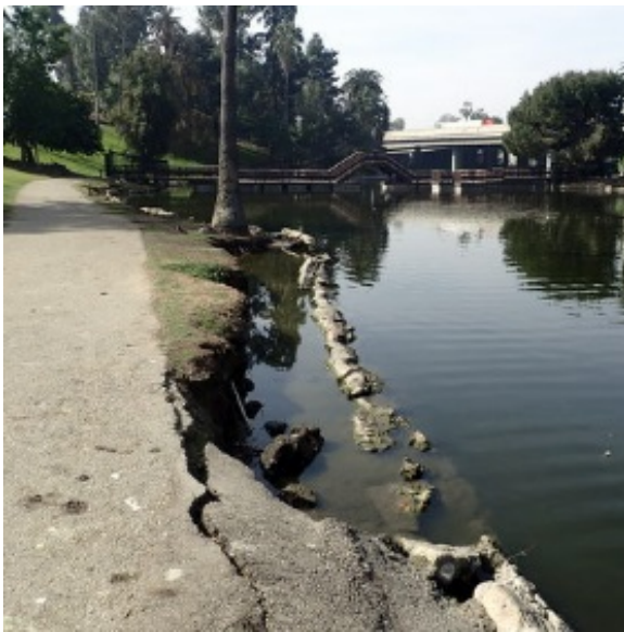
Figure 2-7-I. Lakeside Erosion Undermining Pavement and Tree Hollenbeck Park Lake Rehabilitation and Stormwater Management
