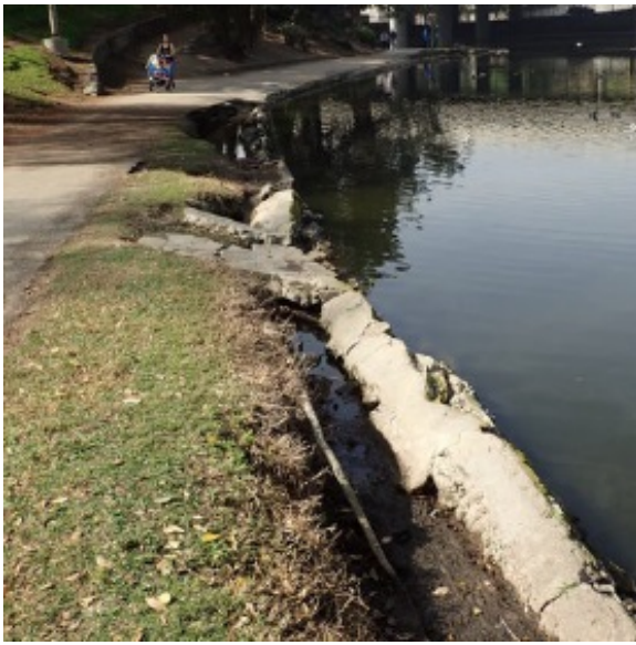
Figure 2-7-K. Lakeside Erosion Exposing Irrigation Lines Hollenbeck Park Lake Rehabilitation and Stormwater Management
