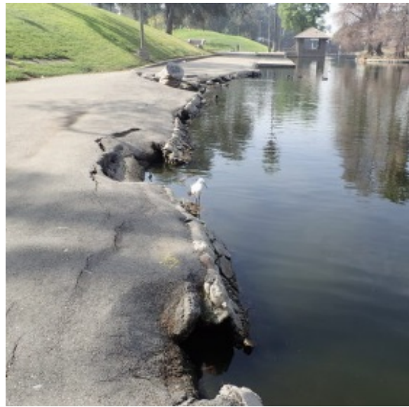
Figure 2-7-H. Lakeside Erosion Undermining Pavement Hollenbeck Park Lake Rehabilitation and Stormwater Management
