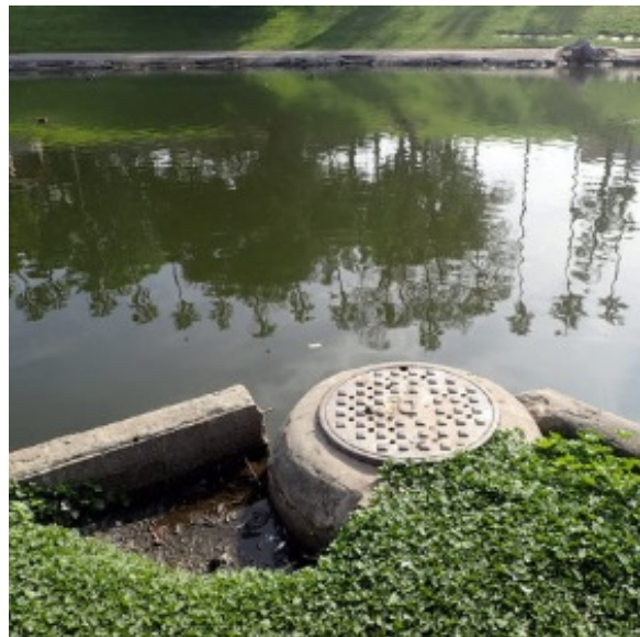
Figure 2-7-F. Lakeside Erosion at Storm Drain Manhole Hollenbeck Park Lake Rehabilitation and Stormwater Management
